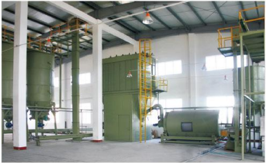
磨粉车间 Mill workshop
