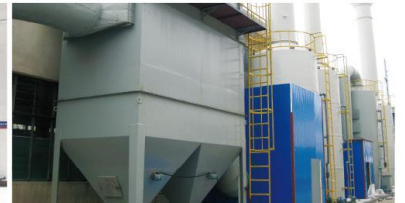
铅尘净化处理系统 Lead dust purification system
