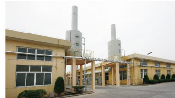
二级酸雾净化塔 Two steps of acid mist purification tower
